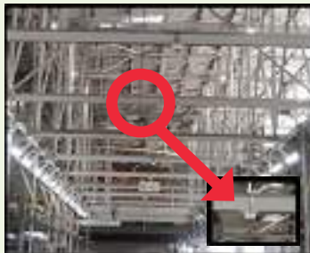
Sensor installed at Cab trim Shop
