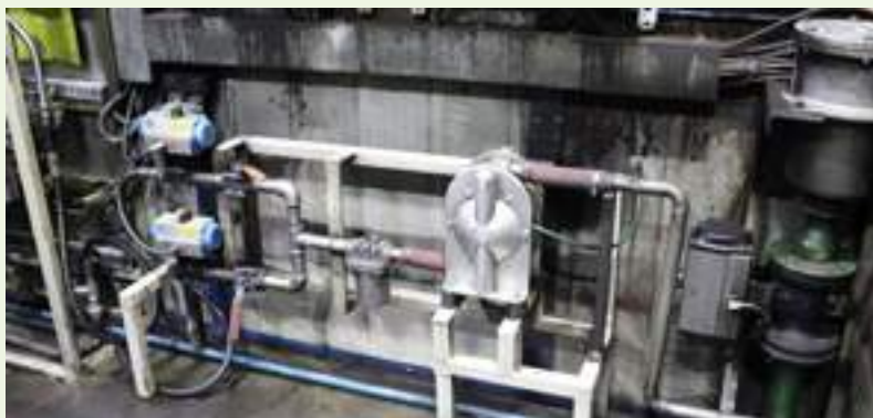
Fuel Drainage System
