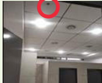
Sensor installed at Office Toilets
