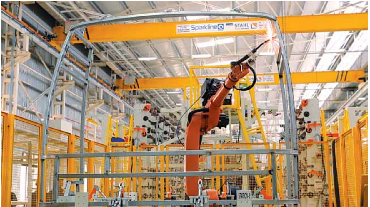
The plant also has robotic welding facilities for main body and under body welding
